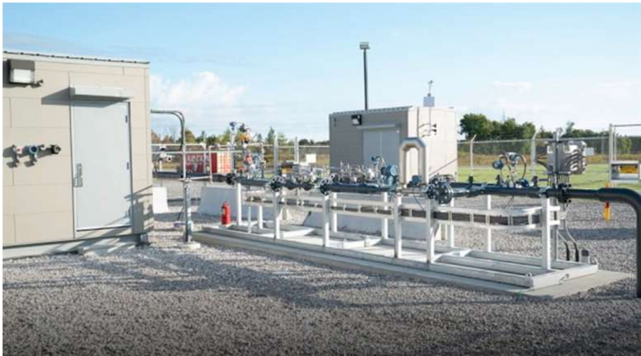
Figure 3-2: Example of a Hydrogen Blend Skid [21]
