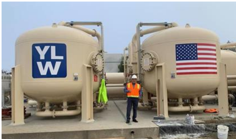
Figure 2: Example anion exchange vessels in a lead/lag configuration (Reproduced from OCWD 2021)
