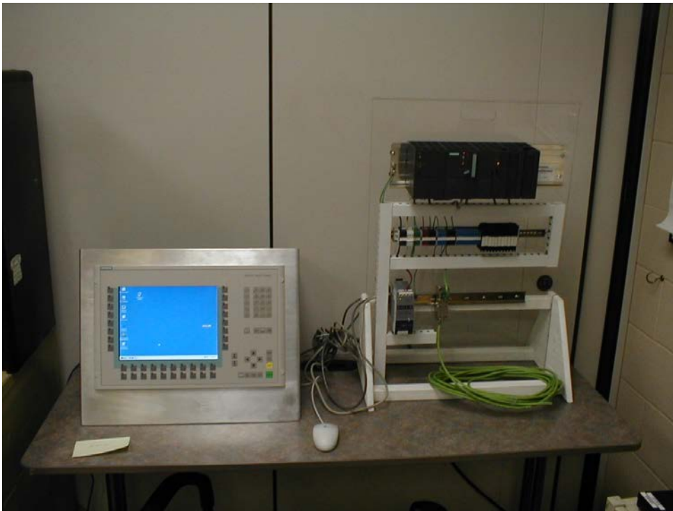
Figure 1. Siemens MP370 Panel and S7000 PLC
