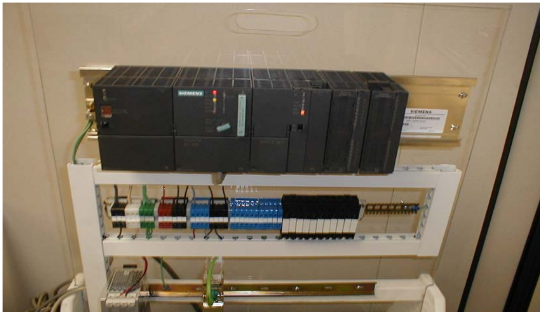
Figure 6. Siemens S7000 PLC
