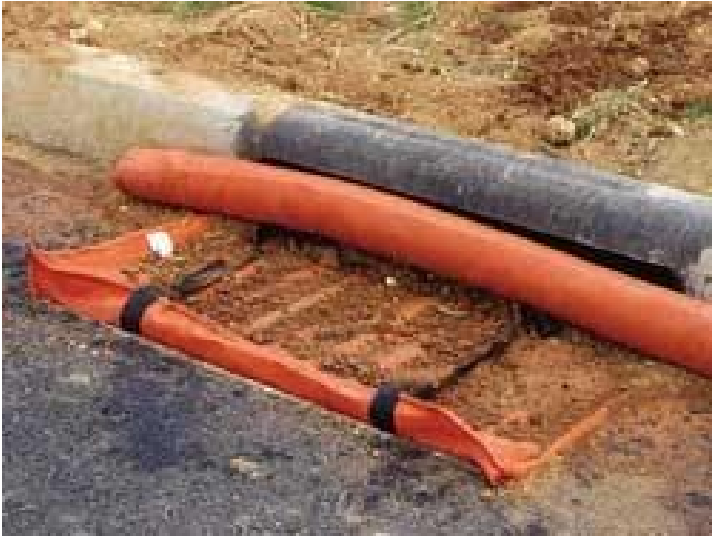
Figure 10.7.1: Temporary Inlet Cover collecting debris
