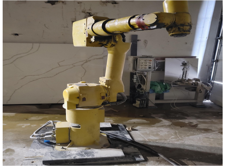
Figure 23: Hooking robot up to electrical
