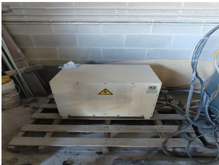
Figure 24: Step up transformer
