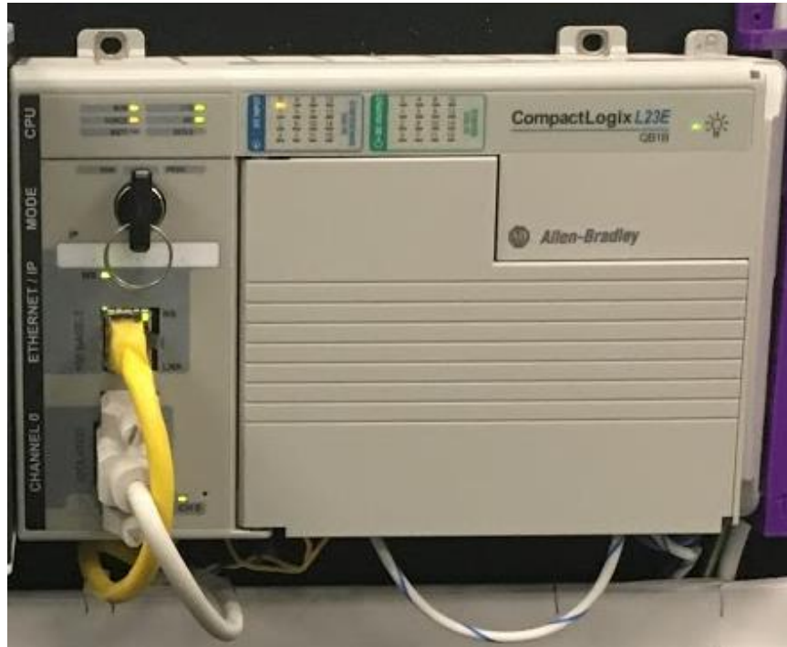
Figure 12: Allen Bradley PLC
