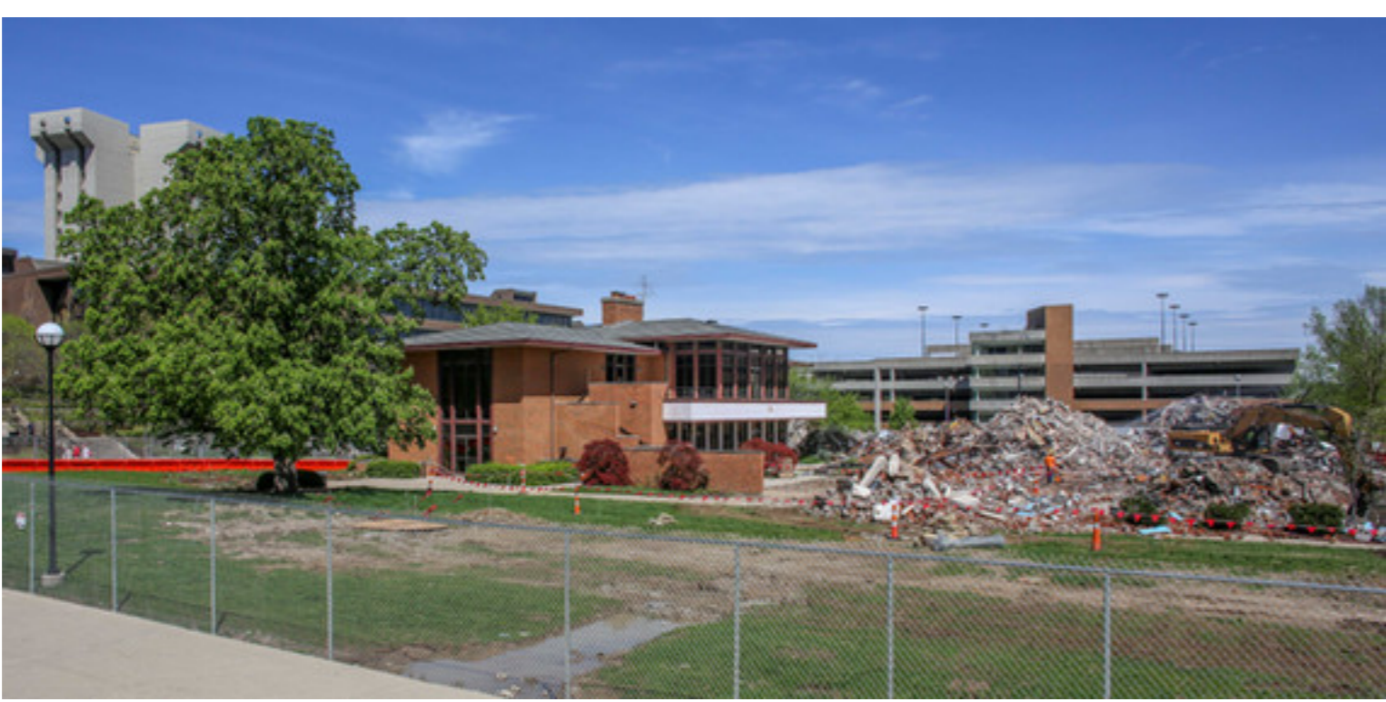
Demolition of University of Cincinnati Faculty - Alumni Center (view from south). 2016. Photograph by Elizabeth Meyer, 2016.
