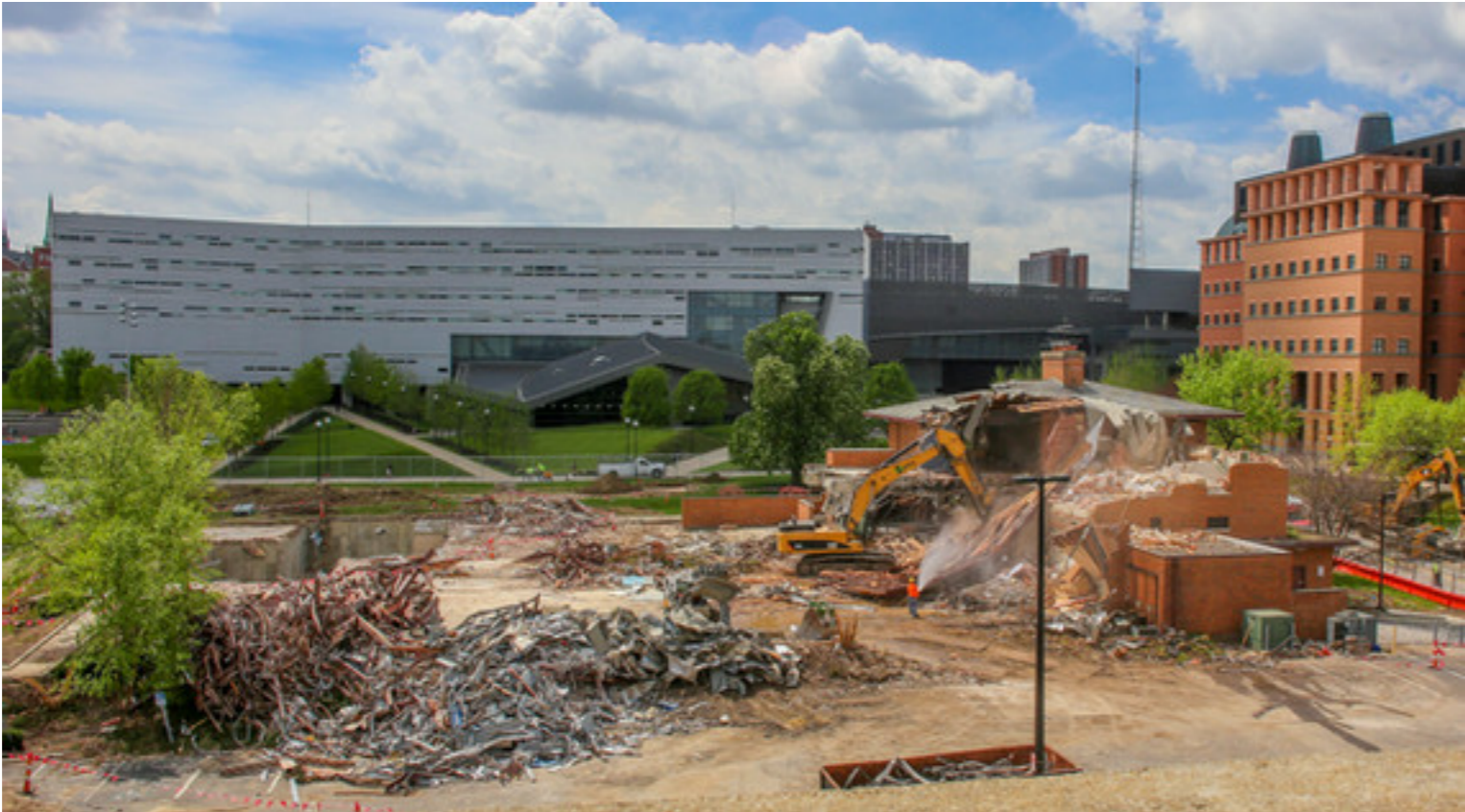
Demolition of University of Cincinnati Faculty - Alumni Center (view from north). 2016. Photograph by Elizabeth Meyer, 2016.
