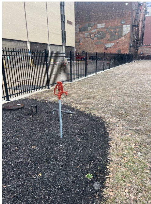
Image showing existing water pump on site.
