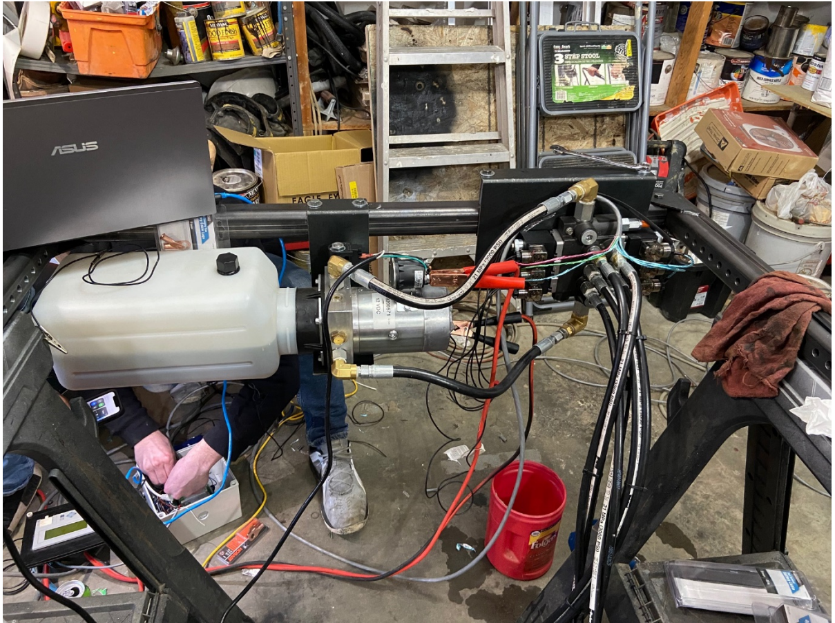
Fig. 12: Hydraulic Pump and Valve Pack
