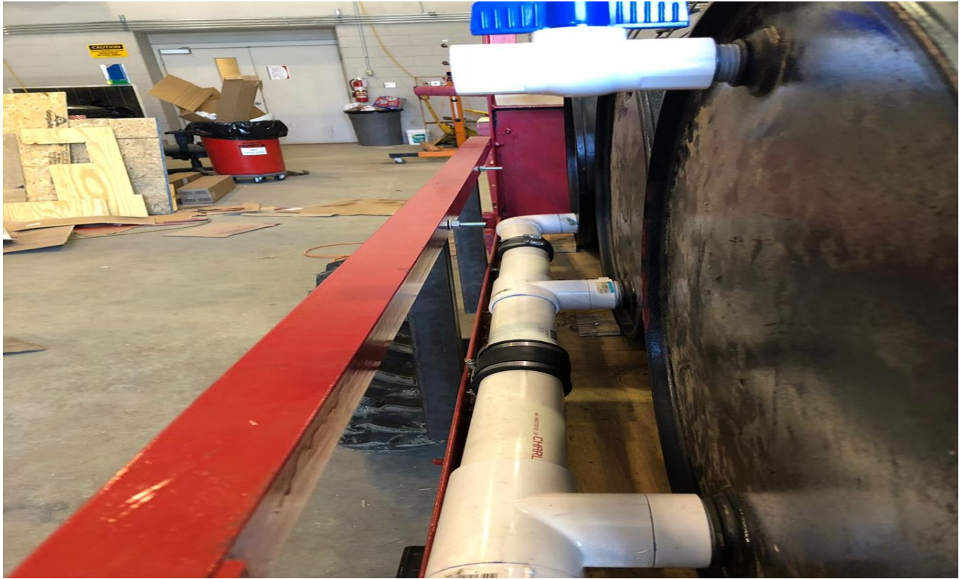
Figure 6 Connection of PVC to barrels
