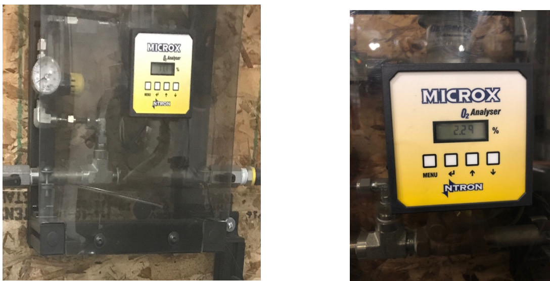
Figure 1.22. the image on the left and right shows the oxygen analyser on the nitrogen generator. This device displays the amount of oxygen that is contained in the main line, the lower the number the better. If the oxygen is low that means the system is running at a higher purity level. The image on the left is before the system was implemented the line contained 17.3% oxygen (82.7 % purity level). The image on the right is after the system was implemented the line contained 2.29% oxygen (97.69% purity level).
