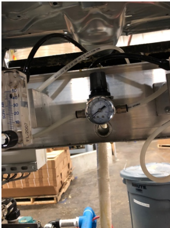
Figure 1.24. shows flowmeter and regulator mounted to the bracket. The bracket is mounted to one of the totes.
