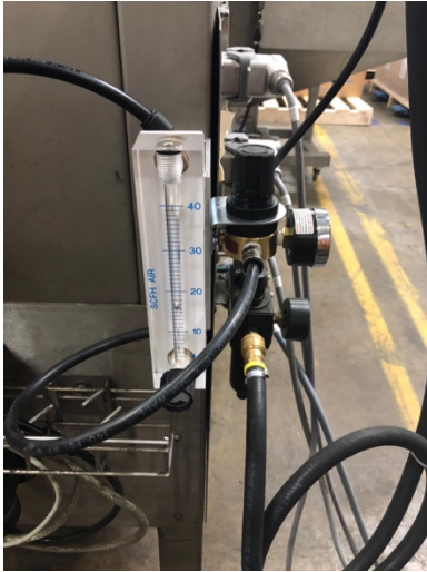
Figure 1.23. shows flowmeter and regulator mounted to the bracket. The bracket is mounted to one of the filling lines.
