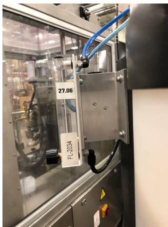
Figure 1.25. shows flowmeter and regulator mounted to the bracket. The bracket is mounted to one of the day-tanks.
