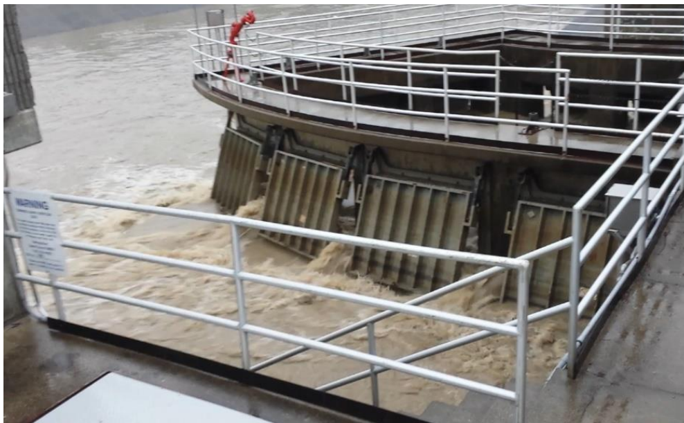
Figure 10. CSO 5 discharging into Mill Creek (CSOs, SSOs, and Sewer Backups n.d.)
