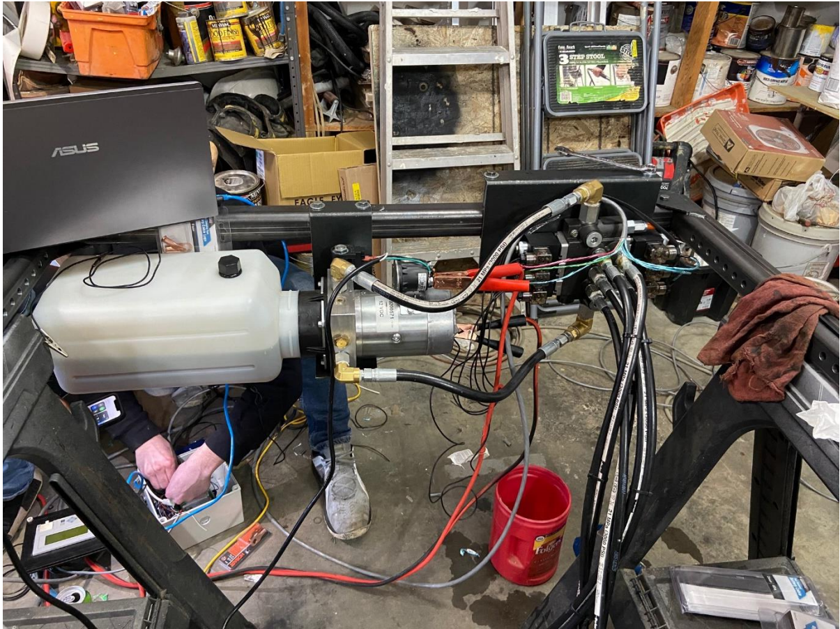
Fig. 9: Hydraulic Pump and Valve Pack, With PLC and HMI (On Floor)
