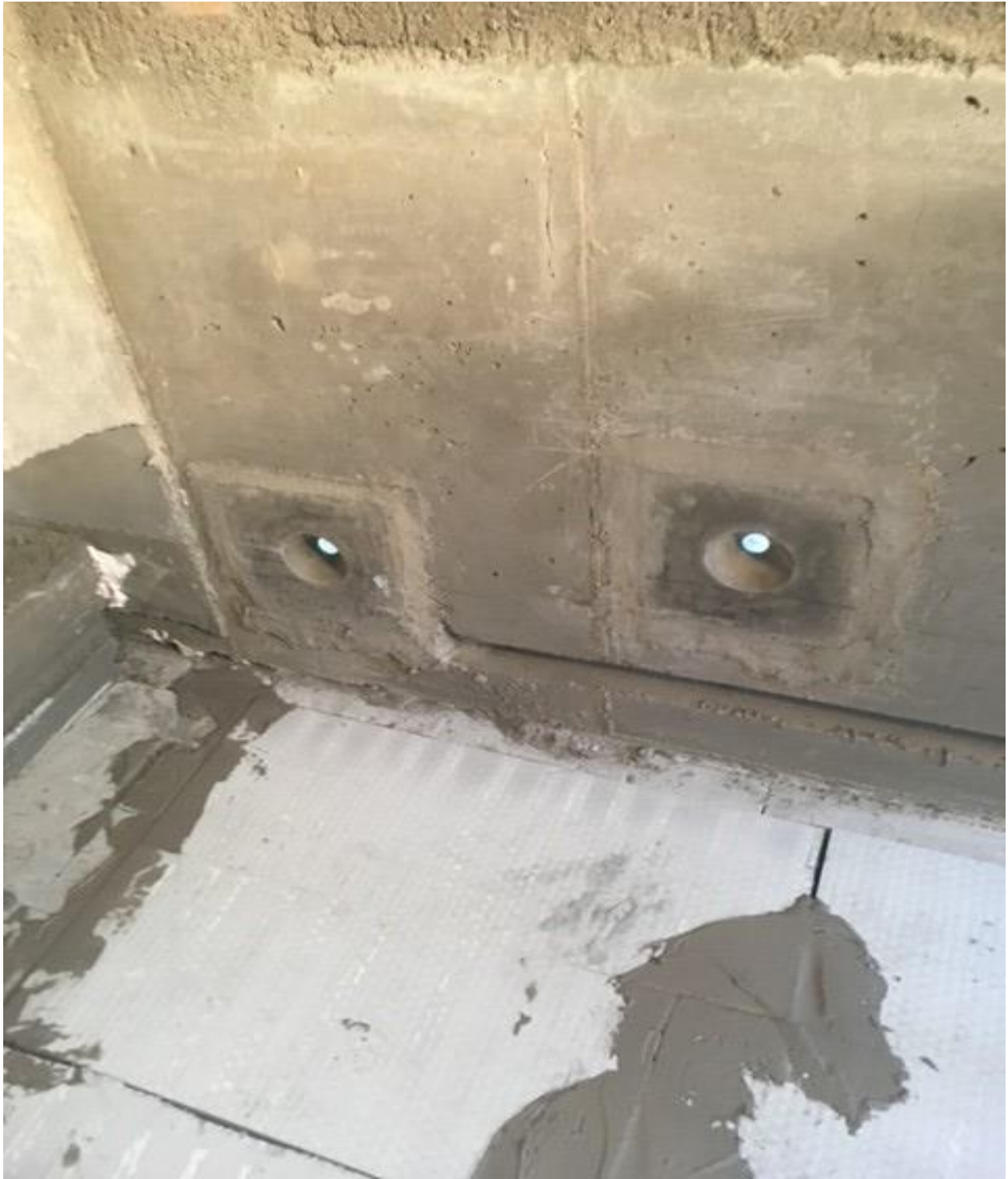
Figure 27 shows the drains from the inside of the holder.
